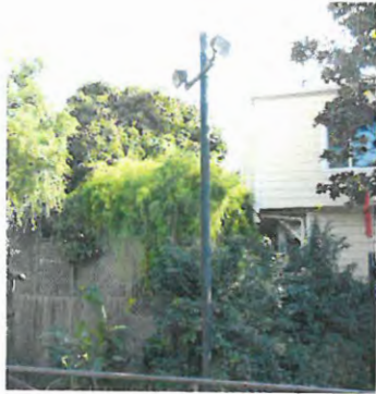
New Light Fixtures
