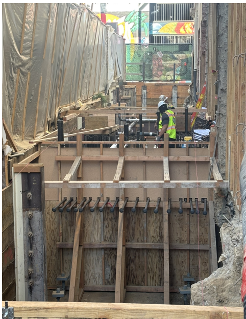
Exterior view from Bartlett St. looking towards Orange Alley — Structural and foundation work. This part of the library is adjacent to a residential building on Bartlett St.
